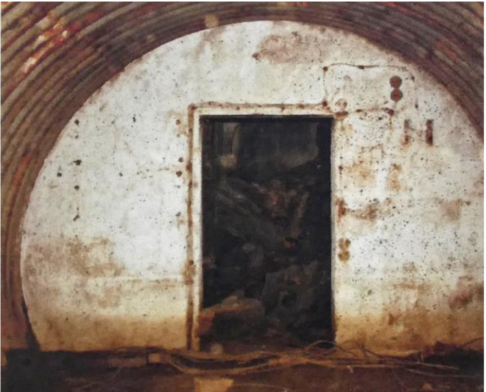
Interior of the Wakehurst Place Zero Station in 2009, it is now unsafe to enter.
