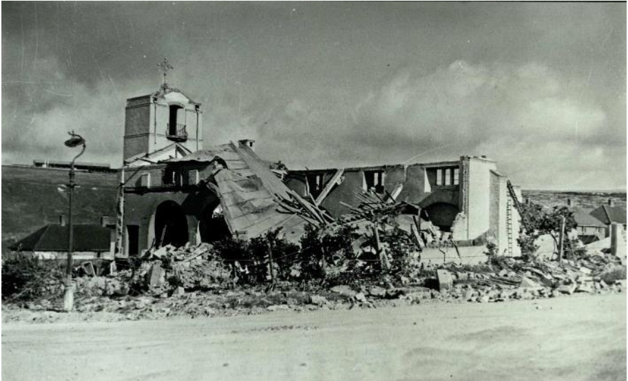
St Cuthman's Church with collapsed roof. © Brighton & Hove RPML
